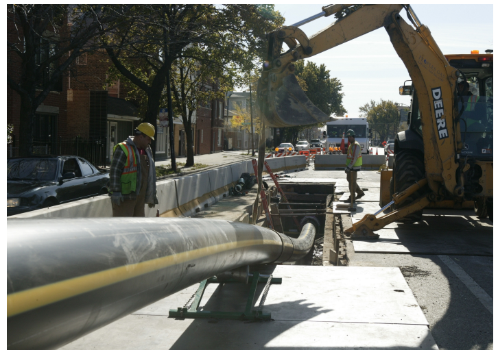
A long, monolithic string of HDPE pipe is threaded under a busy Chicago street as part of the Peoples Gas pipeline replacement program. The driving force was the need for a cost-effective rehabilitation of older cast-iron pipelines.
